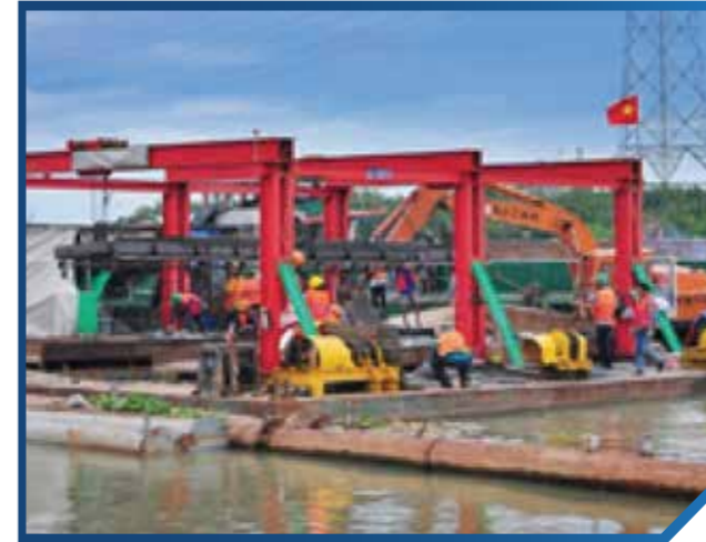
Equipment: Stone carpet machine Origin: Vietnam Quantity: 04 Function: Stone carpet to reinforce the riverbed
