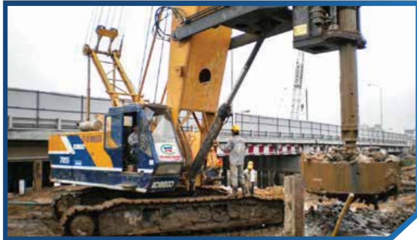
Equipment: D12ED Drilling Rig Origin: Japan Quantity: 04
