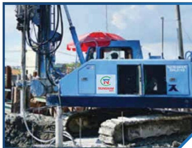
Equipment: XMD Piling Rig Origin: Japan - China - Quantity: 04 Function: Drilling, excavating, and cutting rock for foundations
