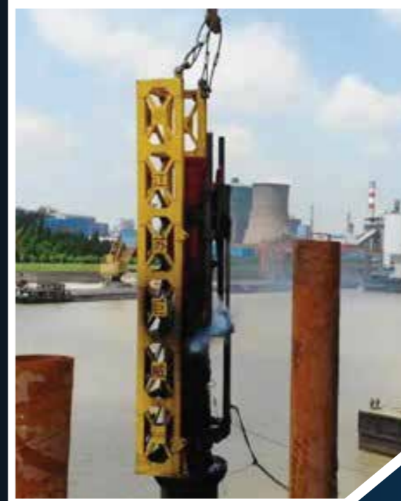
Equipment: 2.5T Diesel Hammer Origin: China Quantity: 06 Function: Driving DUL reinforced concrete D350A piles
